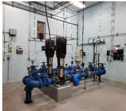
PUMPS FILL THE WATER TANK
